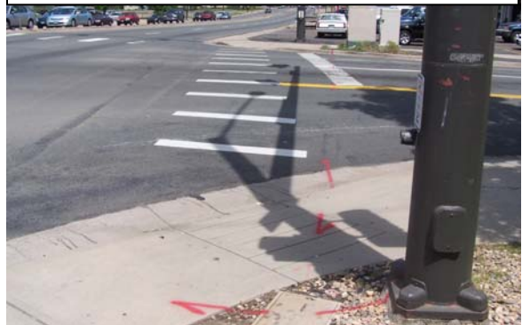
Non-ADA curb ramp at southeast corner of 10 th Avenue/Wadsworth Boulevard
