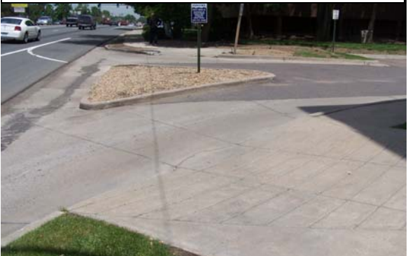
Turn island without curb ramps in pedestrian path (940 Wadsworth Parking Lot Access)
