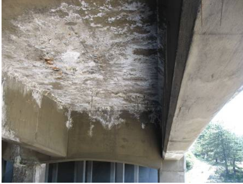
PICTURE 5: EFFLORESCENCE AND RUST ON UNDERSIDE OF DECK
