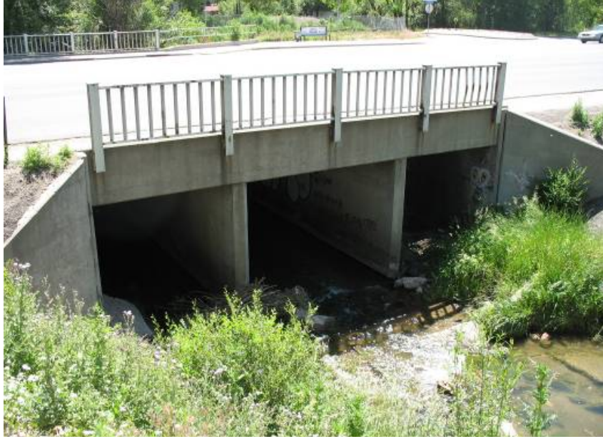
PICTURE 12: BOX CULVERT CARRYING SIXTH AVENUE OVER LAKEWOOD GULCH; WEST SIDE, LOOKING EAST
