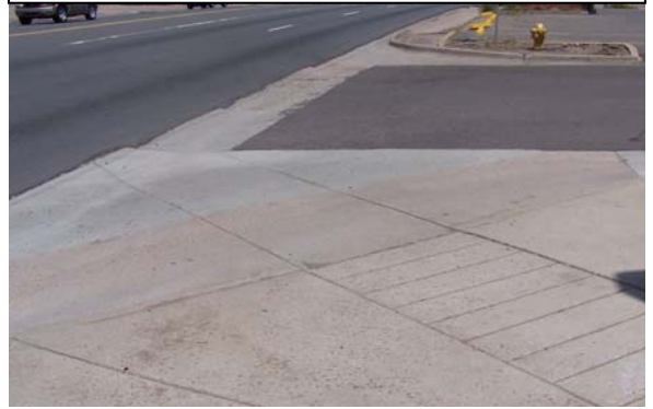
Missing curb ramp on northeast corner of 8 th Place and Wadsworth
