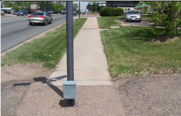
Light Pole obstructing pedestrian traveled way (East side Wadsworth from 6 th to 8 th Avenue)
