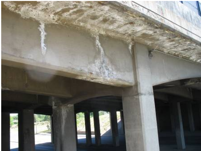
PICTURE 4: OVERHANG OF EASTBOUND BRIDGE
