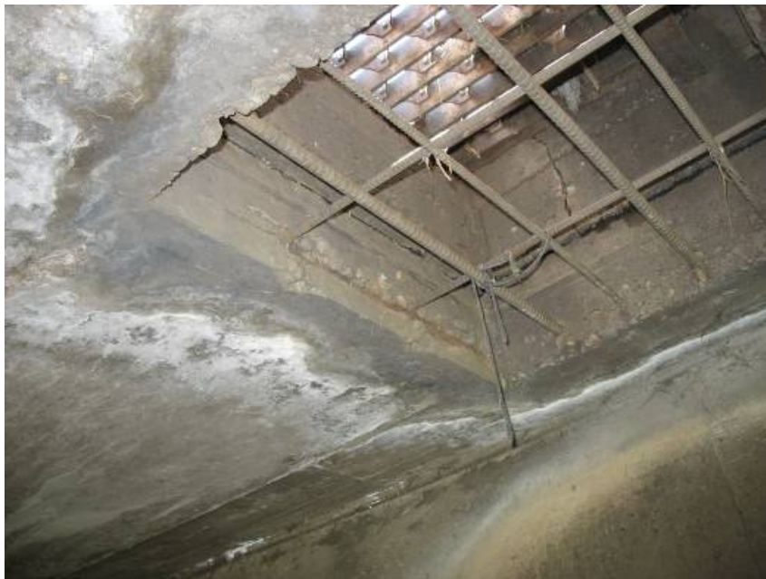
PICTURE 13: BOX CULVERT CARRYING SIXTH AVENUE OVER LAKEWOOD GULCH, TOP SLAB DRAIN
